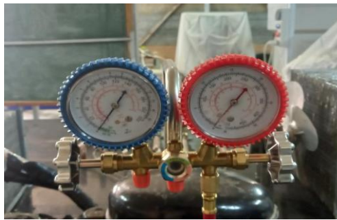
Figure 8: The High and low pressure gauge.
