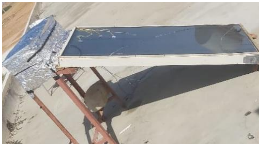
Figure 1: Full experimental solar water heater device operated with thermal pipes.
