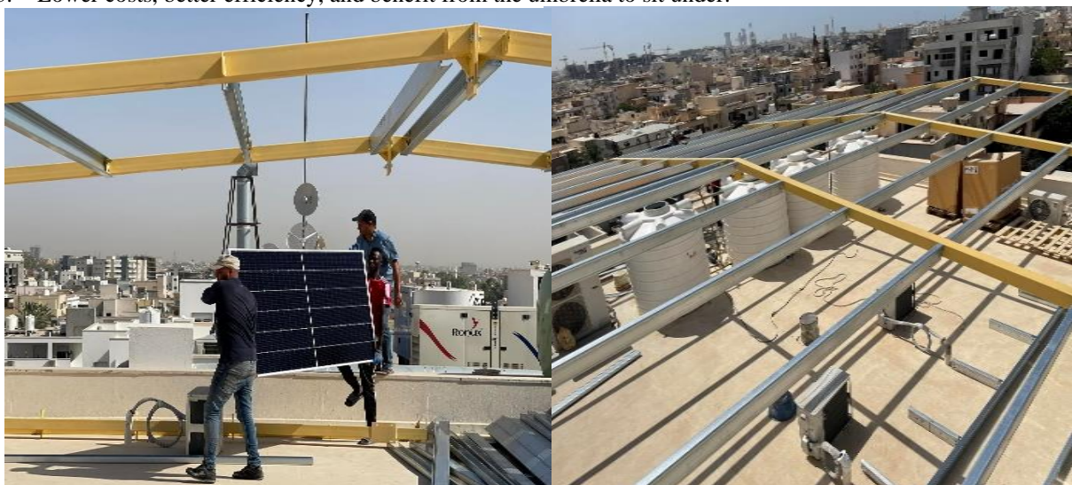
Figure 4 The use of umbrellas on which solar panels are installed [18].
