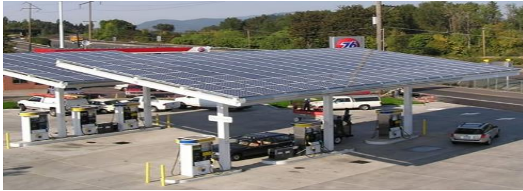
Figure 11 Solar panel Roof, fuel station [26].
