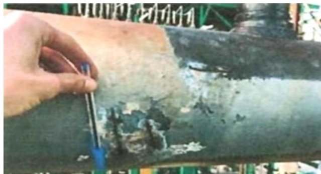
Figure 2: The Shape of the Crack in the Spool Before Cutting.
